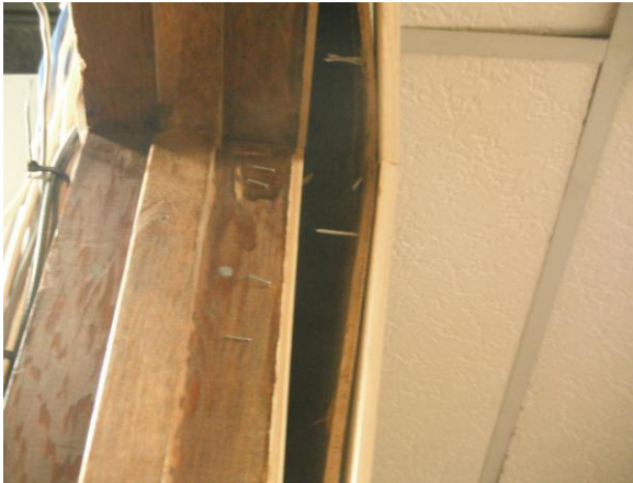
Wall Sheathing Separation 1
