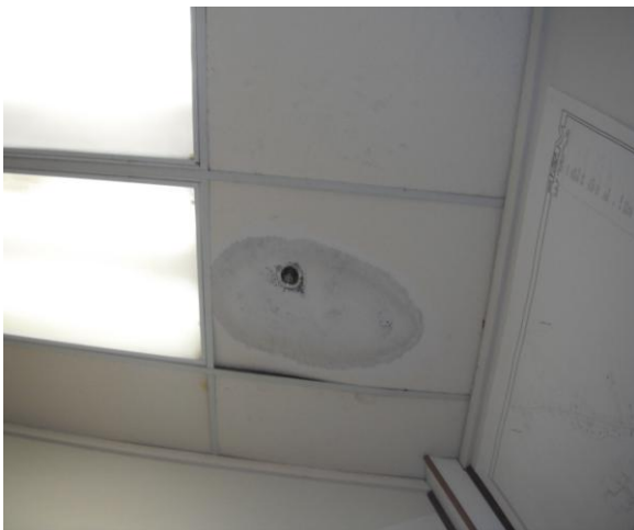
Ceiling Water Damage 1
