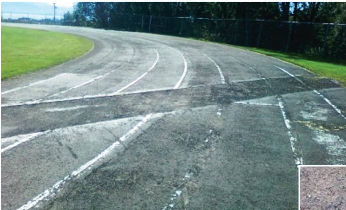
Left: The area of the track that was patched after the 2002 floods is not level.
