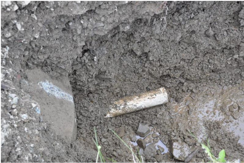
Sewer stub that had no cap on the end of pipe allowing groundwater to run straight in the manhole
