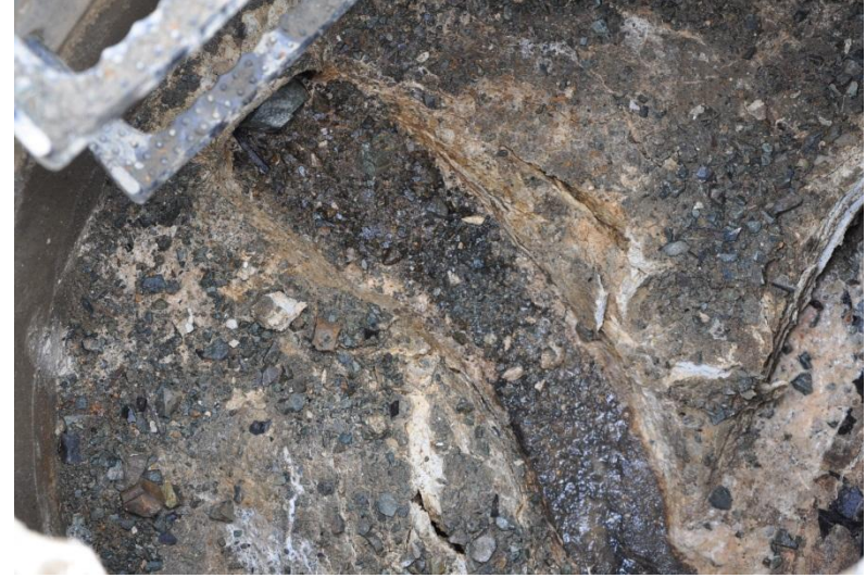
Manhole bottom with concrete flaking away
