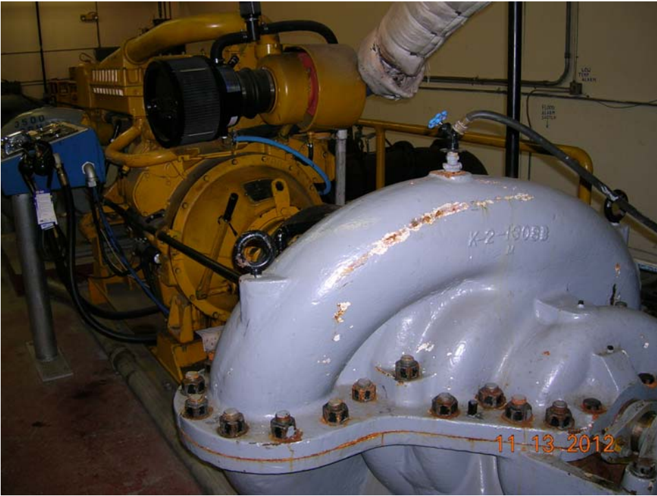
Backup diesel pump
