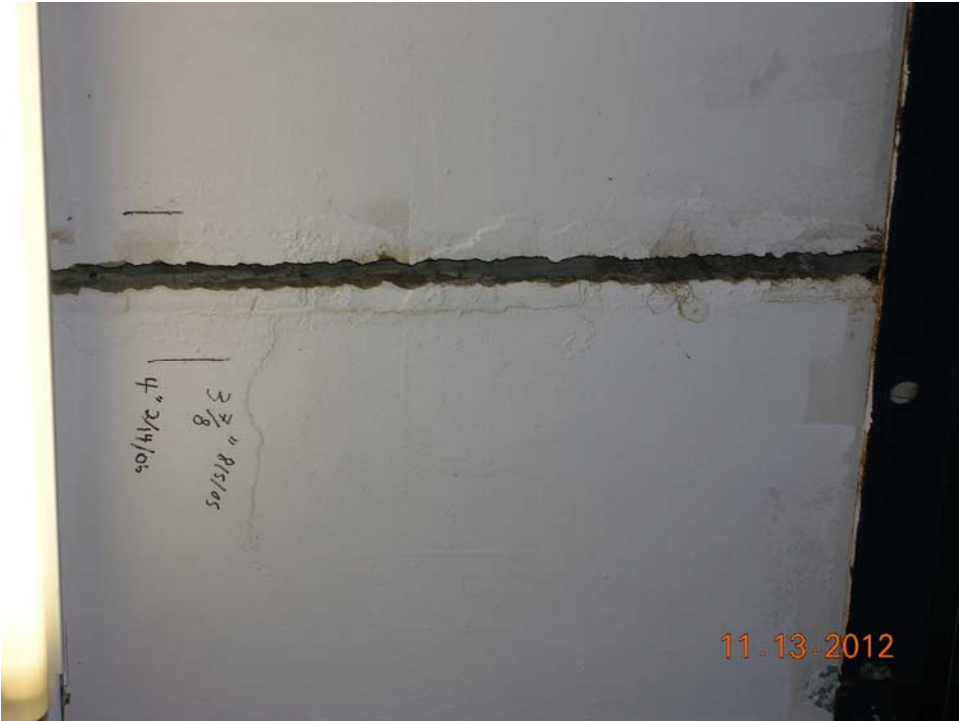
Crack in downstairs ceiling
