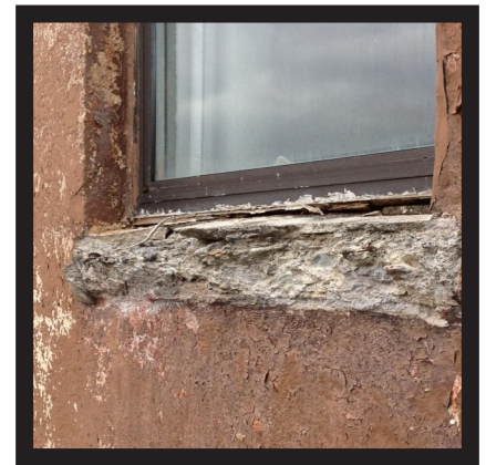
Disintegrating concrete window sill at the Sage Building
