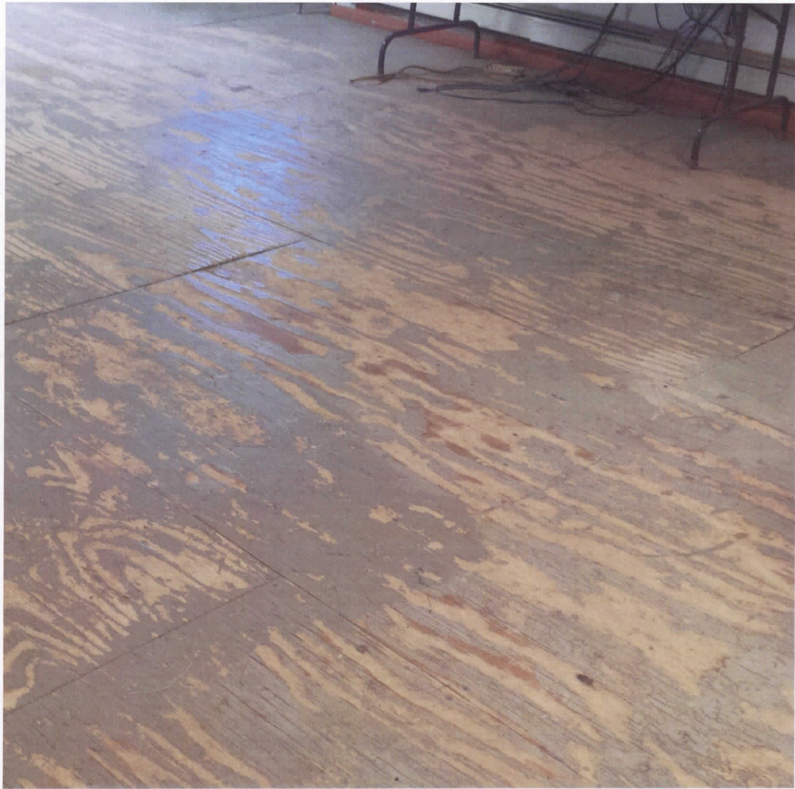
The wood flooring should be replaced with a linoleum floor which will be more resistant to muddy and wet boots.
