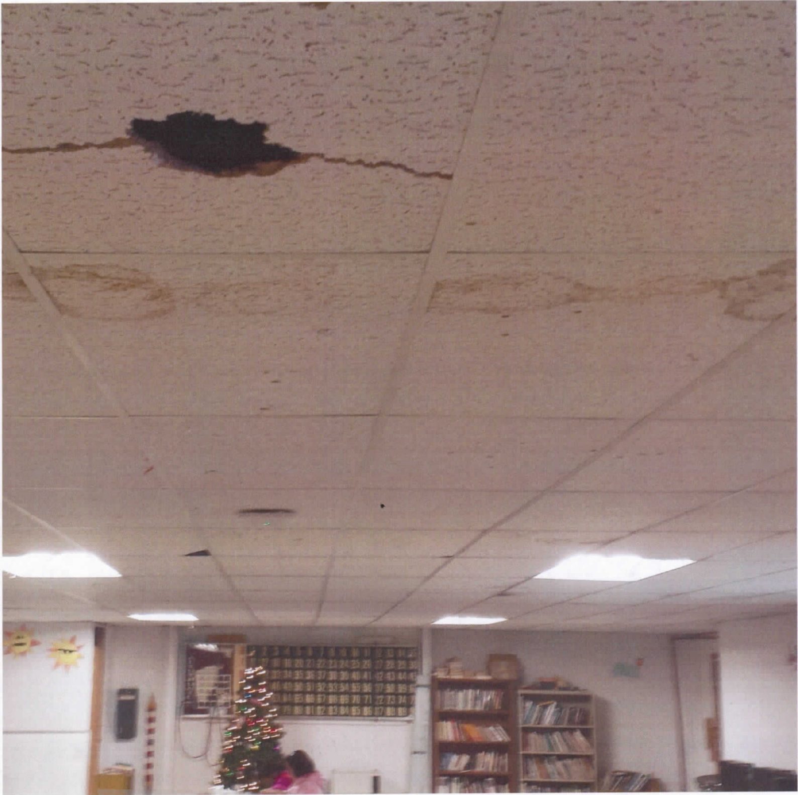
Roof leaks saturate the ceiling tiles, causing them to fall apart.
