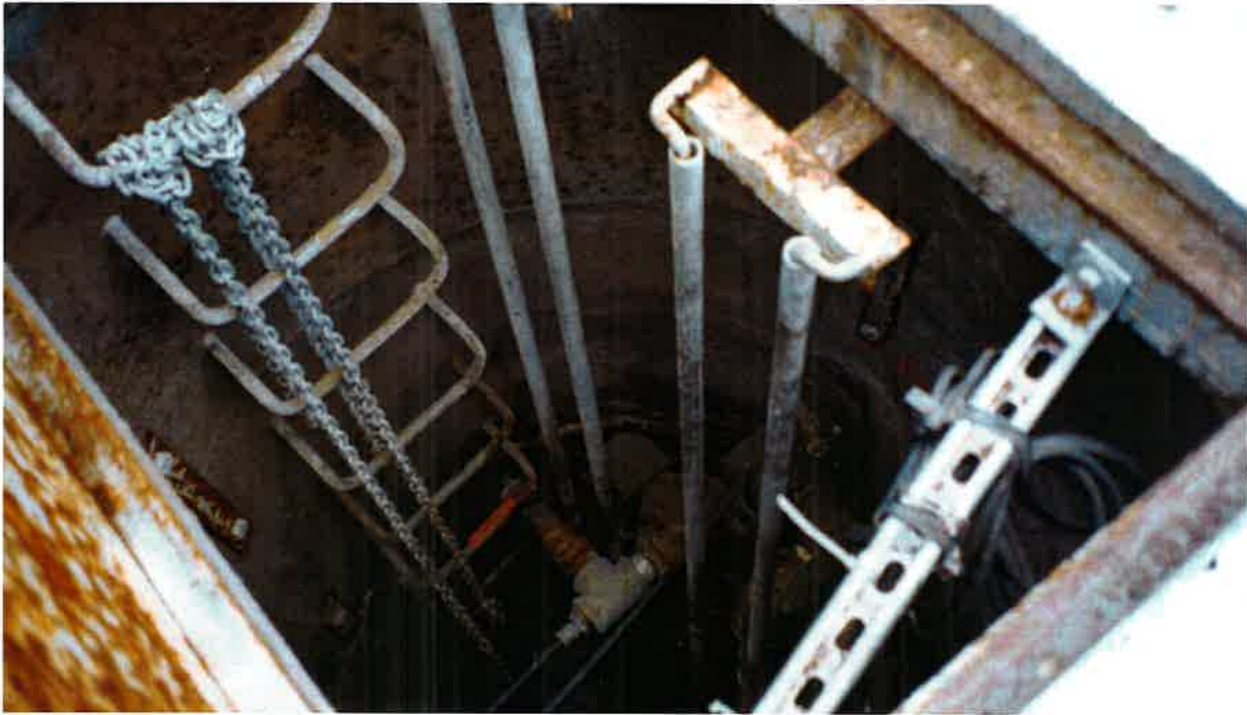
Photo 27. Lift station interior, 6/15/00.
